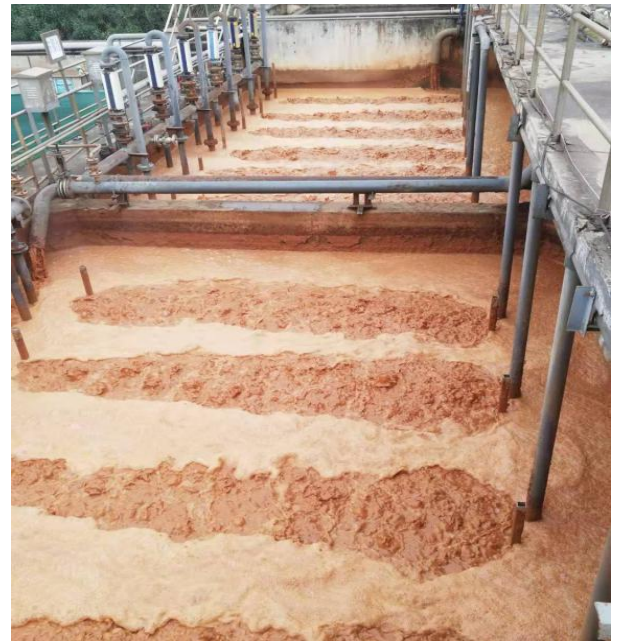
Flat membrane operation after transformation
